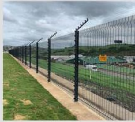
Clear View - fence / security fence and gates
